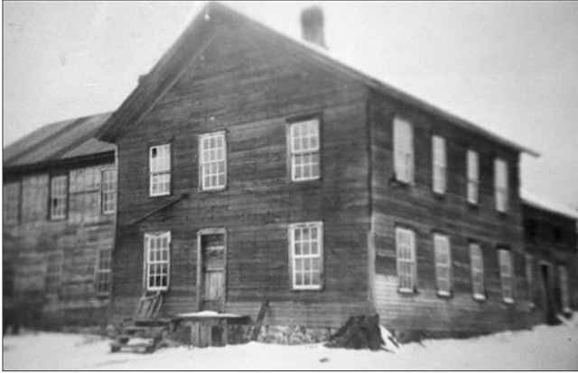
FIGURE 8. The Jayville Hotel at a later time than the previous figure. The porch is gone, a few panes of glass are missing and the cement foundation is exposed. Gerald Miller (Fig. 9) played in the hotel ruins as a boy. Perhaps the sled propped against the lower left window belonged to him. Photo courtesy of Joseph St.Amand, Jr.
