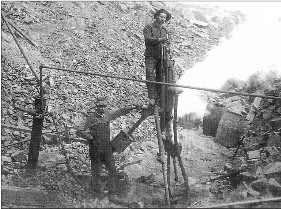
FIGURE 4. Drilling blasting holes in magnetite-bearing bedrock at Benson Mines. The stern-faced man stands on a drill mounted on an iron tripod. A jet of steam used to power the drill is being ejected from a round opening, just below the horizontal pipe. Three wooden barrels lie in the background. Photo by Henry Beach, ca. 1911. From R. Bogden, 2003, p. 138.
