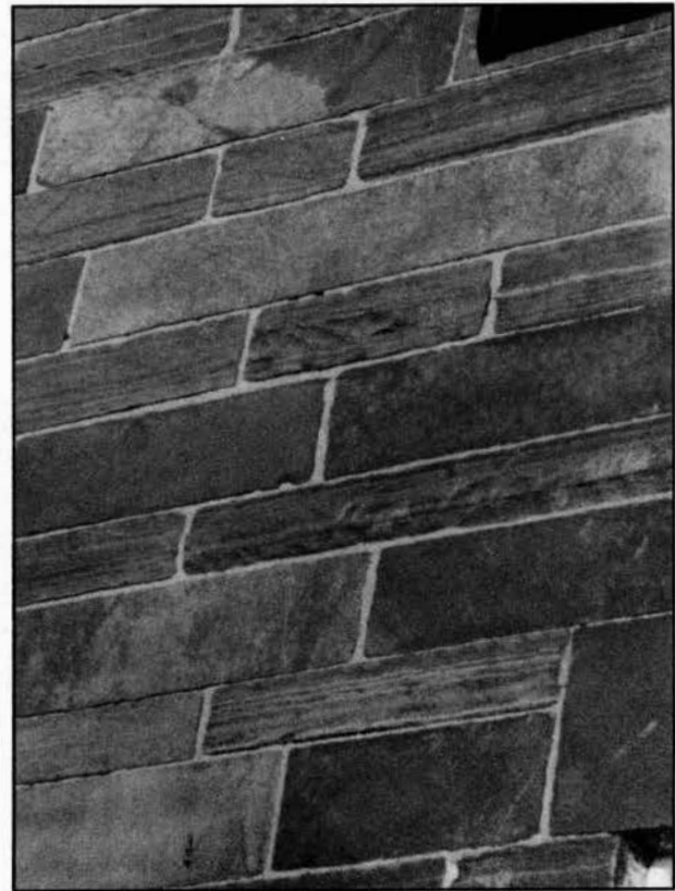
This close view shows the alternating layers of slab and binder masonry
