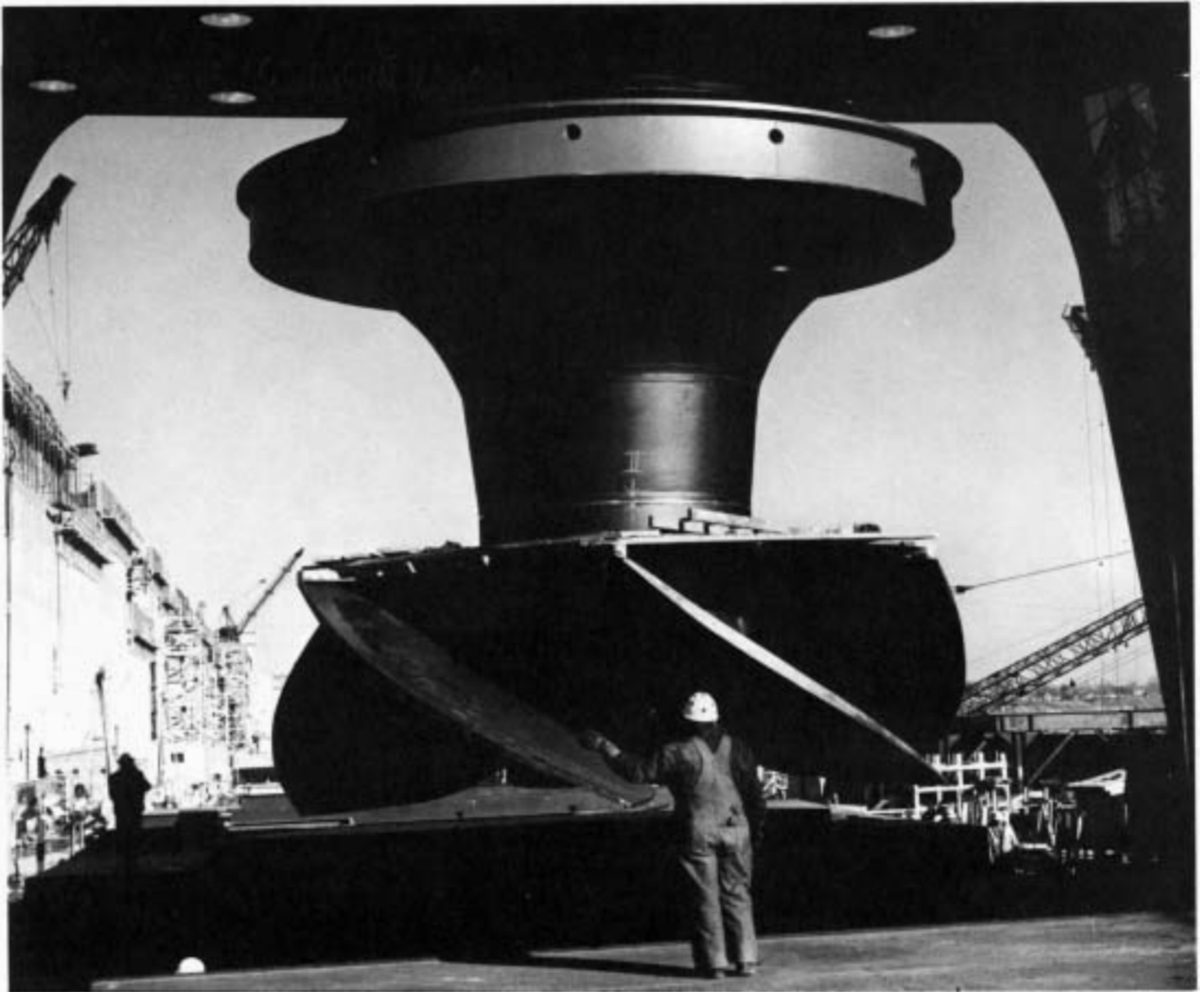
The 150-ton runner assembly is being lowered into position for Unit 30, St. Lawrence Power Dam, on December 17, 1957. (Photograph: Power Authority of the State of New York, courtesy of Nick J. Podgurski)
