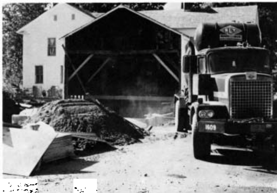
Work underway on addition to museum, June 1986. (Photograph courtesy of the St. Lawrence County Historical Association archives)
