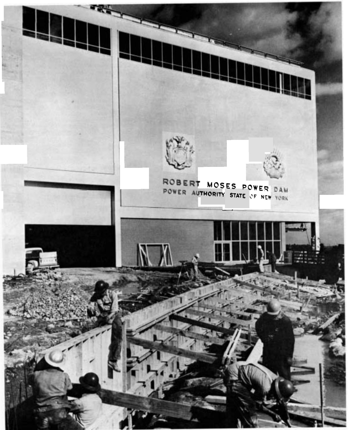
Retaining walls and curbs are being built in the parking area in front of the entrance plaza at the Robert Moses Power Dam. (Photo courtesy of the Dumas family of Massena)
