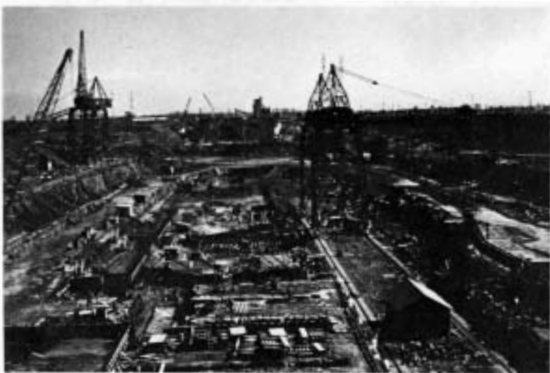
Construction of the Seaway in Massena area. (Photo courtesy of the Dumas family of Massena)
