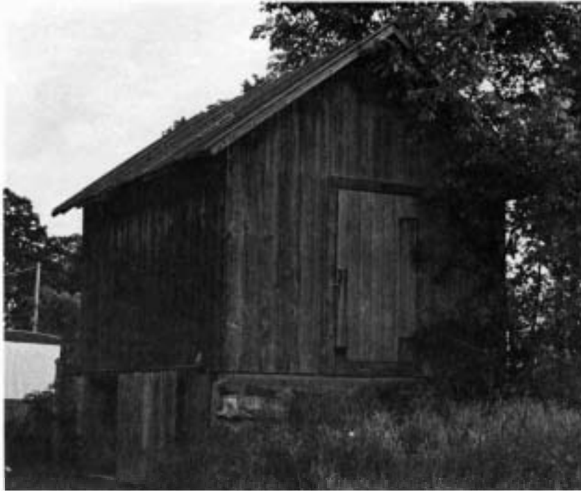
Abandoned granary (upper portion), Rte. 58, Gouverneur. Owner unknown.
