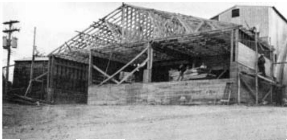
Addition for new wood chipper completed in 1981. (Photo courtesy of the author)
