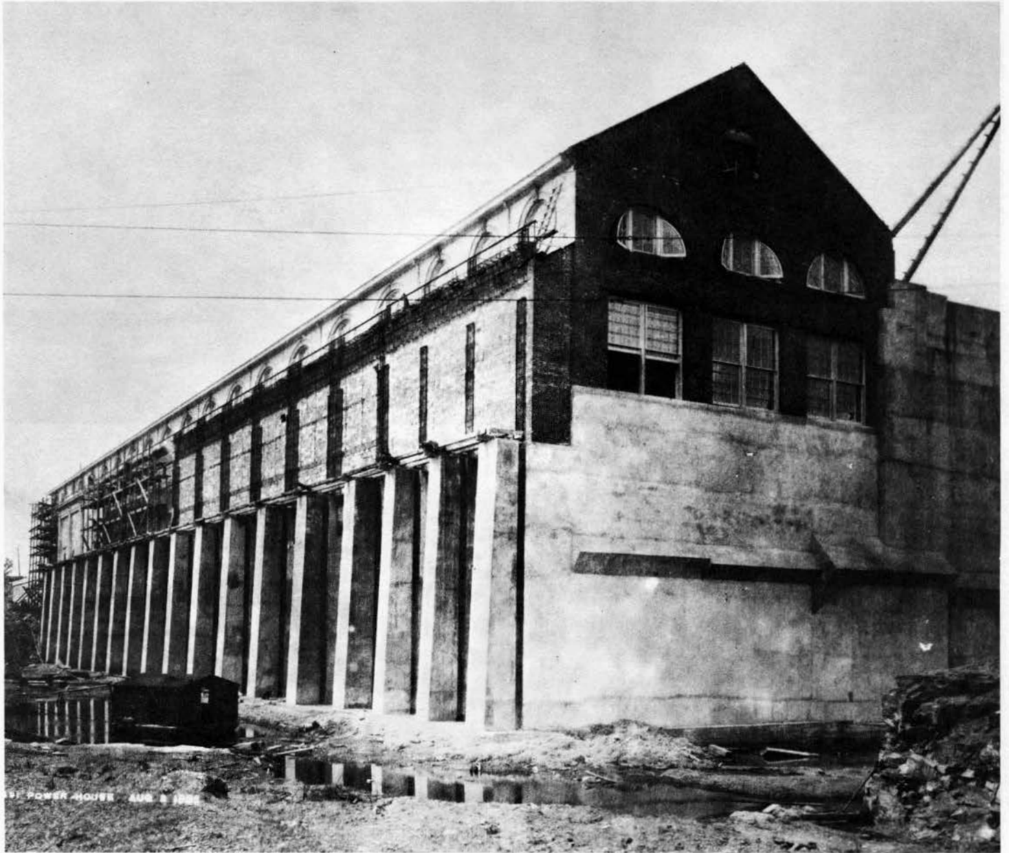
Alcoa's Powerhouse on the Grasse River near completion. Work was begun in 1898 on the power canal, and the canal and powerhouse were completed in 1903 to produce Massena's first metal.
