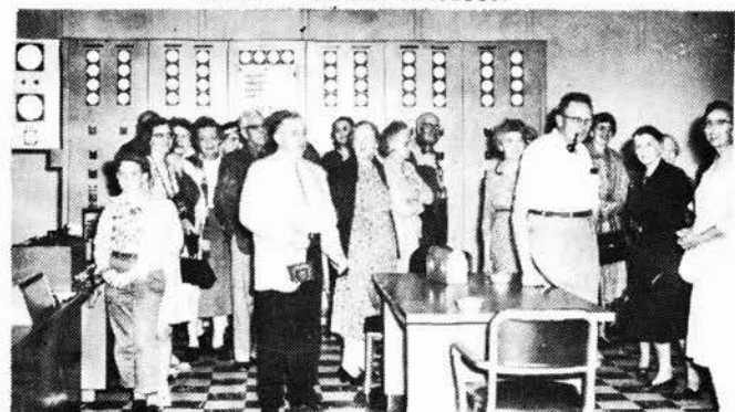
The control station at Colton houses the control center of all the five dams and also controls all of the transmission lines to Northern New York.
